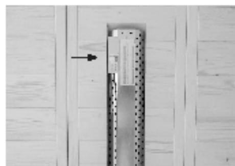
Connection box, top
